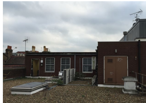
VIEW FROM THE ROOF OF THE BUILDING LOOKING BACK TOWARDS THE BUILDING
